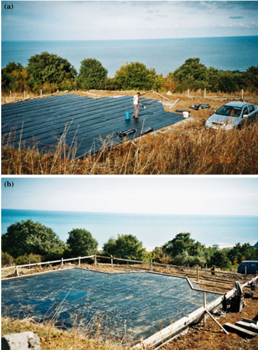
Fig. 3.5 First natural seismic isolated (NSI) private building in Turkey/Samsun (Incesu Mah. Sirincak Sok. No: 2/1) a Preparation of the friction interface—Level 1 b Preparation of the friction interface—Level 2 c General view of building—SN direction d General view of building—NS direction
